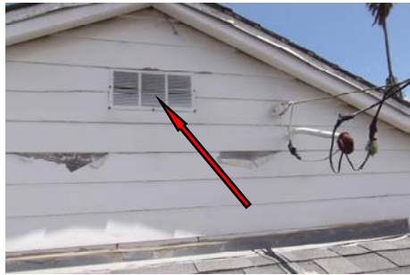
Only Attic Vent
