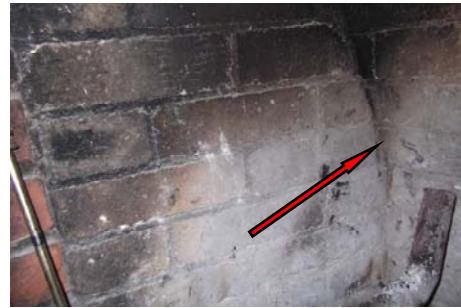
Crack In Left Corner Of Firebox
