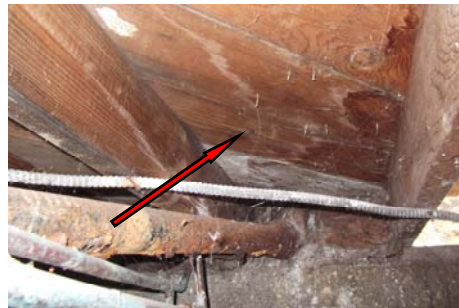
No Insulation Under Floor, Water Damage Observed
