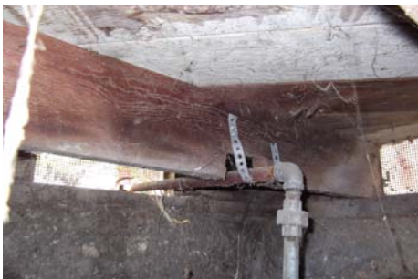
Notch in Floor Joist
