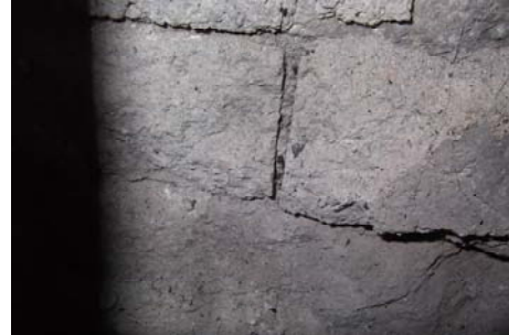
Deteriorating Mortar In Firebox
