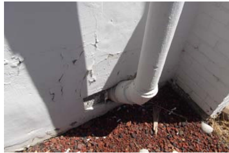
“Asbestos” Like Material, Unused Flue Pipe
