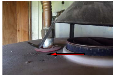
Improper Position Draft Diverter, Exhaust Spill Observed
