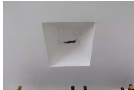
Abandoned Exhaust Vent
