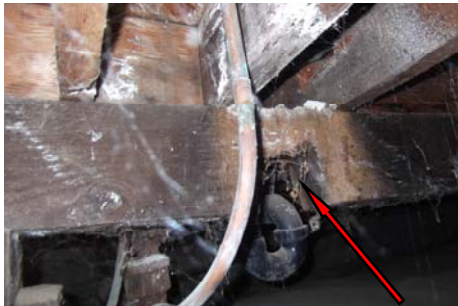
Notching in Girder
