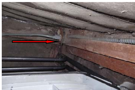
Suspect Garage Electrical
