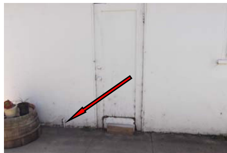
Un-insulated Gas Pipe In Concrete
