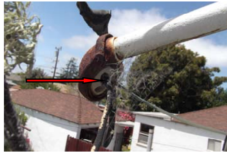
Frayed Service Wires
