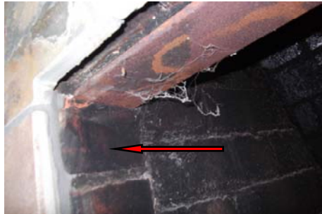
Evidence of Poor Draft
