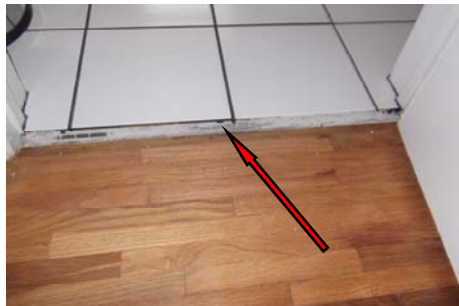
Missing Threshold Piece
