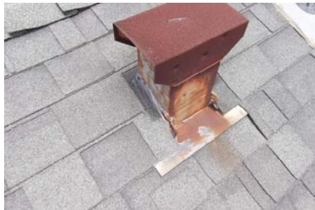
Rusted Abandoned Exhaust Vent
