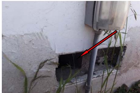
Damaged Vent Screen
