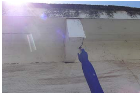
Detached Garage Eave Rot
