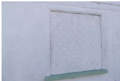
Boarded Up Window
