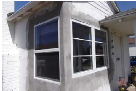
Repair Evident, Monitor For Leaks
