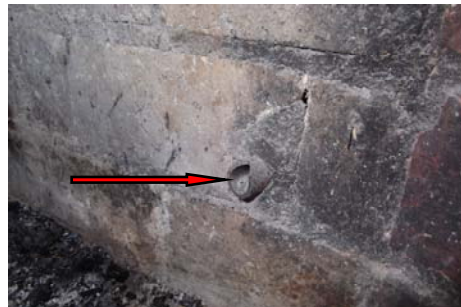
Unsealed Pipe In Firebox
