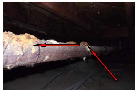
Waste System Deterioration
