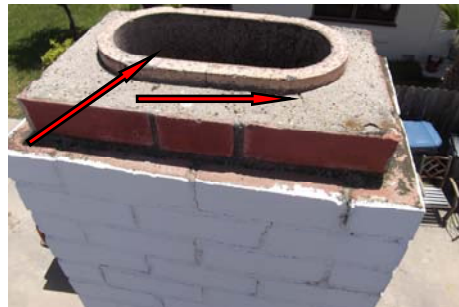
Cracked Crown and Flue Liner, Missing Spark Arrester and Cap
