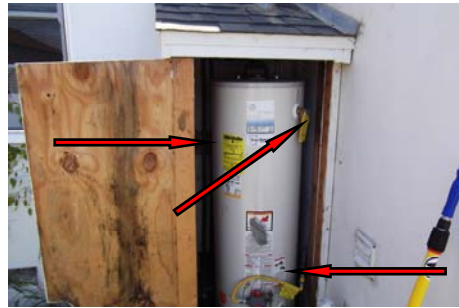
Seismic Straps Needed, Missing TPRV Extension
