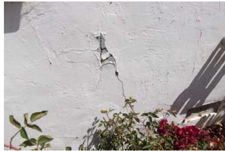
Cracks In Stucco
