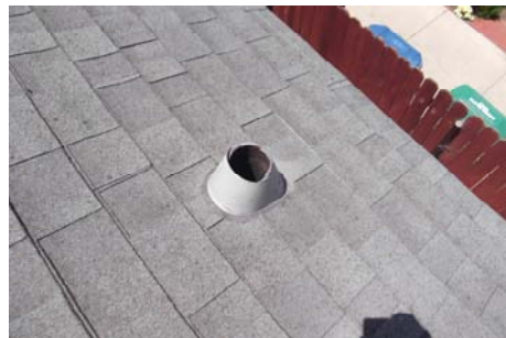
Un-sealed Flashing. Vent Pipe Insufficient Height
