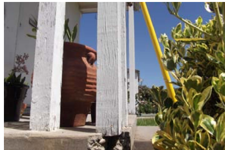
Deteriorated Concrete Under Support
