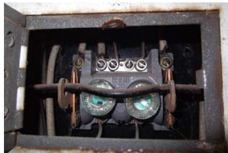
30 Amp Main Fuses
