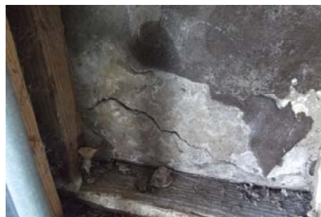
Deteriorated Garage Stucco and Paper, Moisture Damage On Sill
